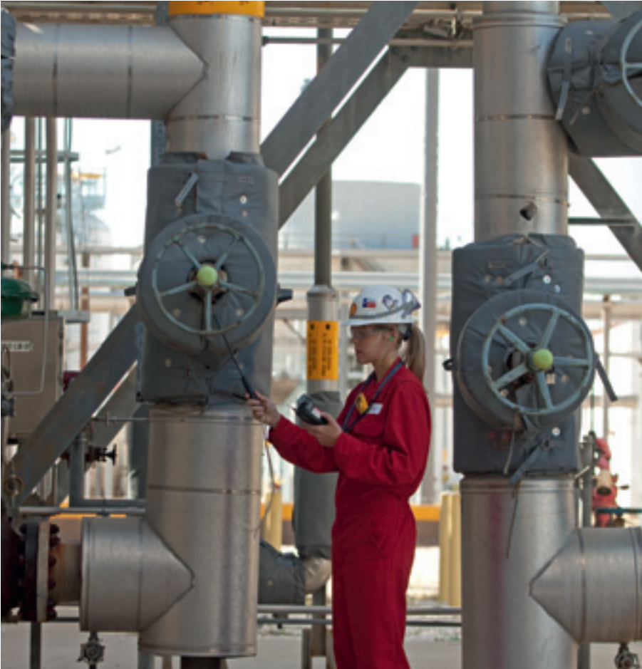
↑ Regular checks help maintain equipment at our Deer Park refinery in Texas, USA.
